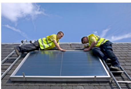
Workmen installing a solar thermal panel on the roof of Pinmore ceramics gallery. They have received advice from the Energy Agency Ayrshire.
